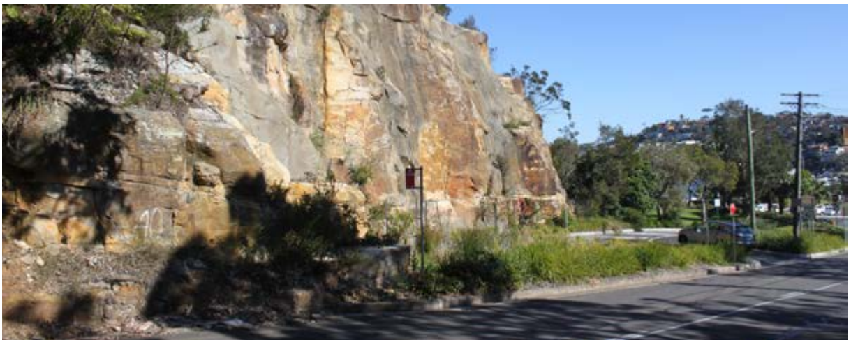
A combination of stable rock with a textured shotcrete applied in minimal areas to stabilise the cutting and provide structural support (The Spit, Sydney)
