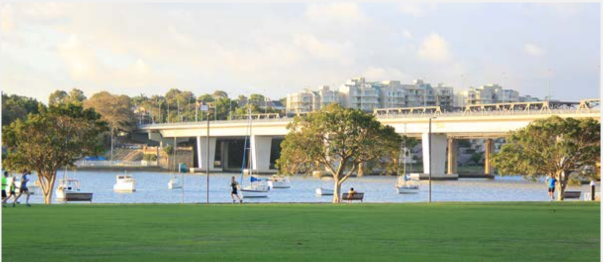
The Bay Run path was realigned and improved, the playground in King Georges Park was used for the project construction site but rebuilt to modern standards. The pontoon used for the project was retained for boating access.
