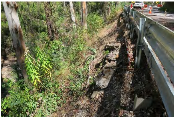
Figure 41. Site 13, intact dry stone wall adjacent to culvert at chainage 30-35m, erosion along embankment, looking south. Source: Extent Heritage, March 2023.
