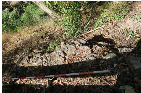
Figure 42. Site 13, intact dry stone wall adjacent to culvert at chainage 30-35m, erosion along embankment, looking east towards Darkey Creeks. Source: Extent Heritage, March 2023.
