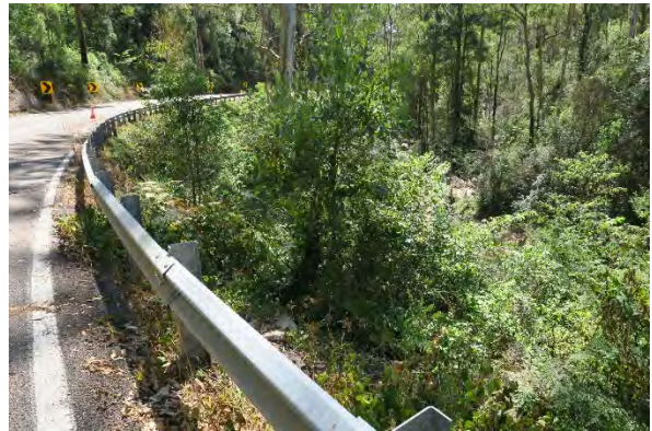
Figure 24. Site 7, loss of embankment with heavy vegetation along steep embankment slope to Darkey Creek, looking north. Source: Extent Heritage, March 2023.
