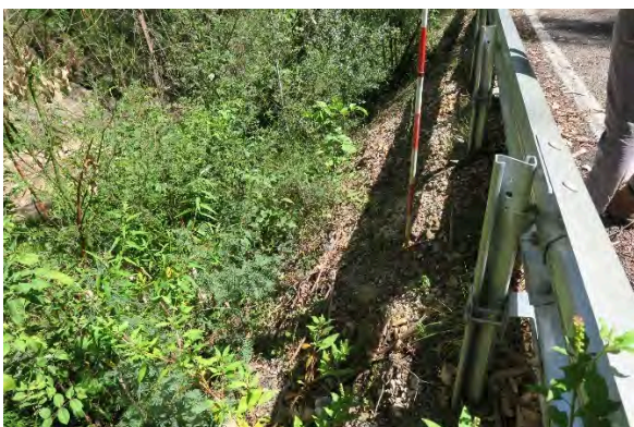
Figure 47. Site 13, embankment loss with erosion and heavy vegetation along steep embankment slope, looking south. Source: Extent Heritage, March 2023.
