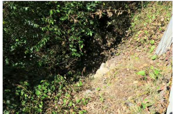
Figure 12. Site 3, eroded slope and vegetation above dry stone headwall, looking down to culvert at chainage 120m. Source: Extent Heritage, March 2023.
