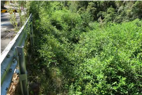
Figure 31. Site 10, embankment loss and heavy vegetation on steep embankment slope towards Darkey Creek, looking north. Source: Extent Heritage, March 2023.
