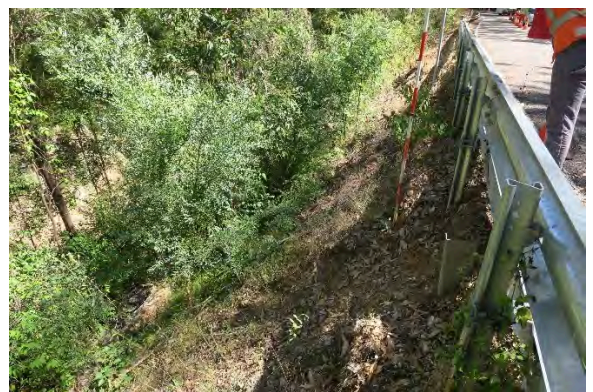
Figure 48. Site 13, embankment loss with erosion and heavy vegetation along steep embankment slope, looking south. Source: Extent Heritage, March 2023.
