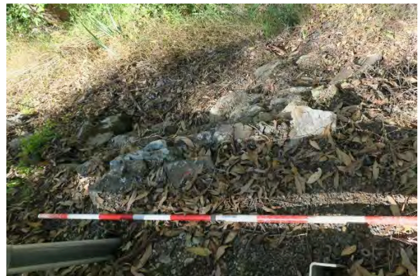
Figure 46. Site 13, detail of dry stone wall at chainage 45-50m, erosion along embankment, looking downslope towards Darkey Creek. Source: Extent Heritage, March 2023.
