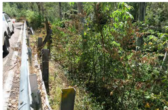
Figure 18. Site 4, embankment loss and heavy vegetation along the steep embankment slope, looking north. Source: Extent Heritage, March 2023.
