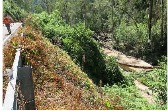
Figure 10. Site 3, embankment loss and heavy vegetation along the steep embankment slope, looking north. Source: Extent Heritage, March 2023.
