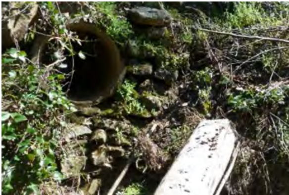
Figure 23. Site 7, detail of culvert and dry stone headwall covered in heavy vegetation. Source: Newcastle Geotech, September 2022.
