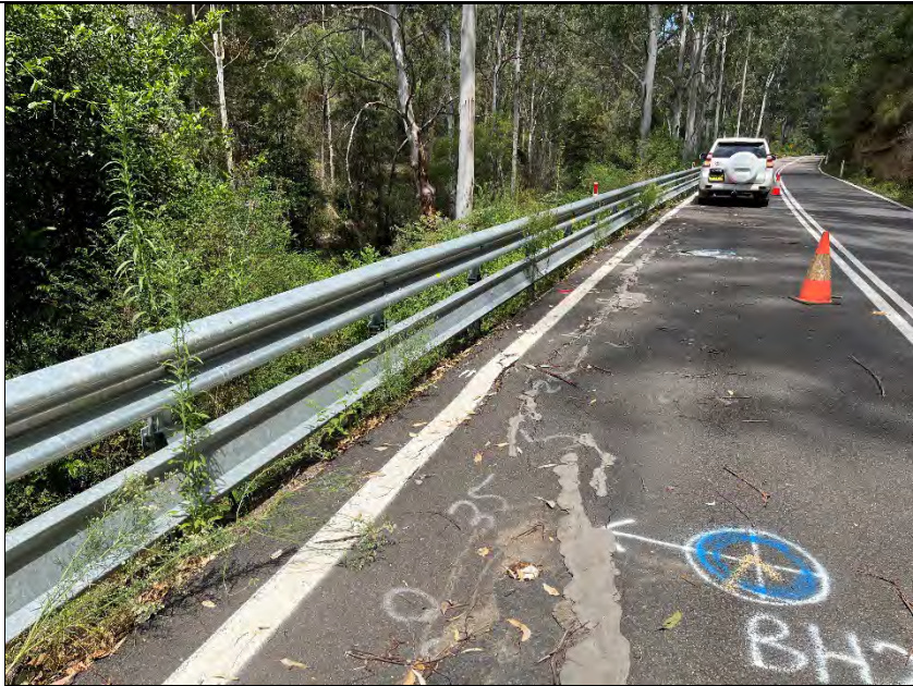
Cracks in road surface caused by slope failure present in study area.
