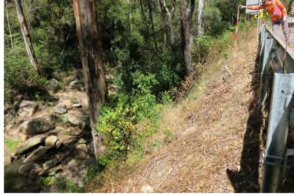
Figure 36. Site 11, erosion and embankment loss downslope with some vegetation towards Darkey Creek, looking south. Source: Extent Heritage, March 2023.
