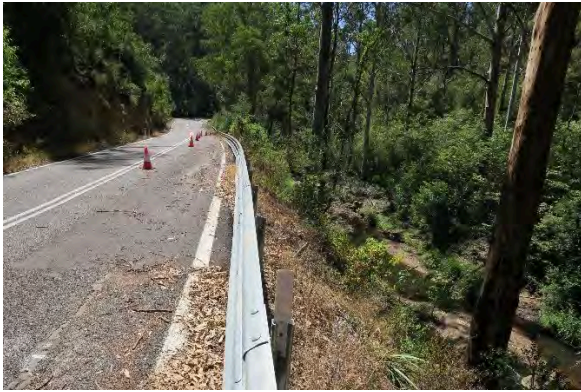
Figure 35. Site 11, erosion and embankment loss downslope towards Darkey Creek, looking north. Source: Extent Heritage, March 2023.
