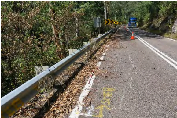
Figure 25. Site 8, steep slope towards Darkey Creek with embankment loss with heavy vegetation, looking south. Adjacent cutaway secured with metal netting. Source: Extent Heritage, March 2023.
