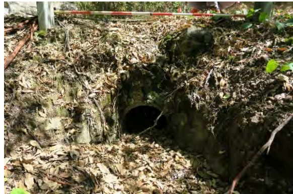
Figure 28. Site 9, culvert 357111 and dry stone headwall with evidence of concrete additions. Source: Extent Heritage, March 2023.
