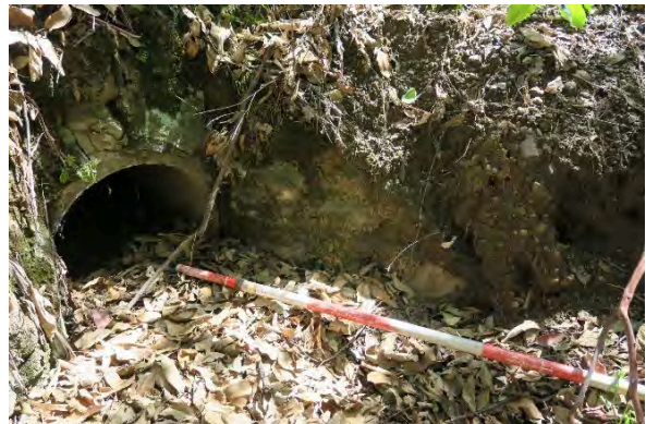
Figure 30. Site 9, detail of culvert 357111 and dry stone headwall with evidence of concrete additions. Source: Extent Heritage, March 2023.
