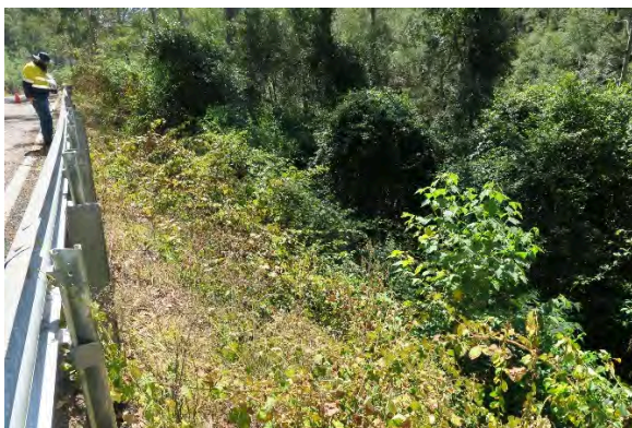
Figure 19. Site 5, embankment loss and heavy vegetation along the embankment slope, with a steep drop off to Darkey Creek, looking north. Source: Extent Heritage, March 2023.
