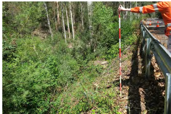
Figure 34. Site 10, embankment loss and heavy vegetation on steep embankment slope towards Darkey Creek, looking south. Source: Extent Heritage, March 2023.
