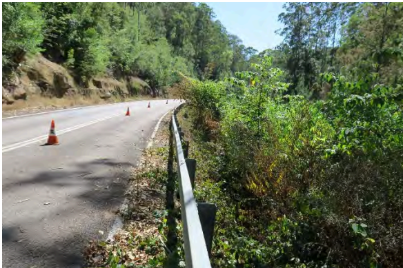
Figure 11. Site 3, embankment loss and heavy vegetation along the steep embankment slope, looking north. Source: Extent Heritage, March 2023.
