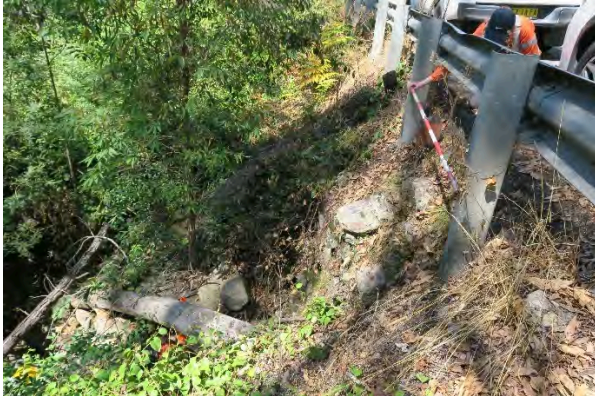
Figure 21. Site 7, eroded dry stone headwall and culvert with 2m scale, looking south. Source: Extent Heritage, March 2023.
