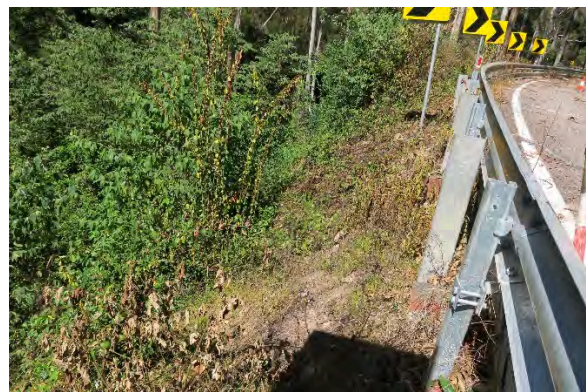
Figure 20. Site 5, embankment loss and heavy vegetation along the embankment slope, with a steep drop off to Darkey Creek, looking south. Source: Extent Heritage, March 2023.
