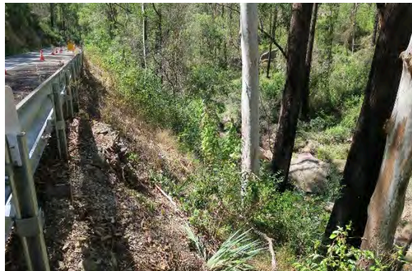
Figure 40. Site 13, intact dry stone wall adjacent to culvert at chainage 30-35m, erosion along embankment, looking north. Source: Extent Heritage, March 2023.
