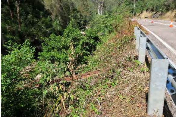
Figure 9. Site 3, embankment loss and heavy vegetation along the steep embankment slope, looking south. Source: Extent Heritage, March 2023.
