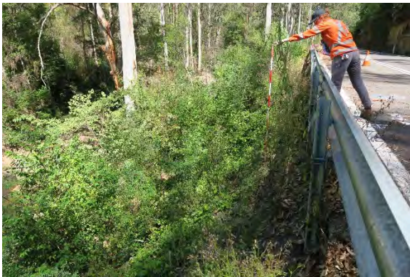
Figure 33. Site 10, embankment loss and heavy vegetation on steep embankment slope towards Darkey Creek, looking south. Source: Extent Heritage, March 2023.
