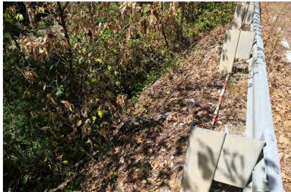
Figure 26. Site 8, erosion and embankment loss with heavy vegetation downslope to Darkey Creek, looking south. Source: Extent Heritage, March 2023.
