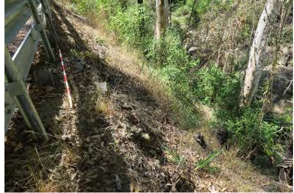
Figure 44. Site 13, dry stone wall at chainage 45-50m, erosion along embankment, looking north. Source: Extent Heritage, March 2023.
