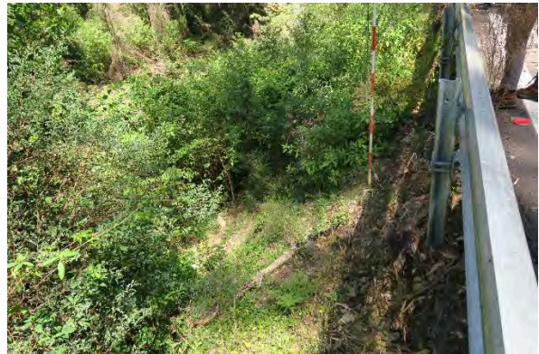
Figure 32. Site 10, embankment loss and heavy vegetation, timber post visible, looking south. Source: Extent Heritage, March 2023.
