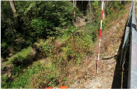
Figure 37. Site 13, erosion and embankment loss downslope towards Darkey Creek, looking slope. Source: Extent Heritage, March 2023.
