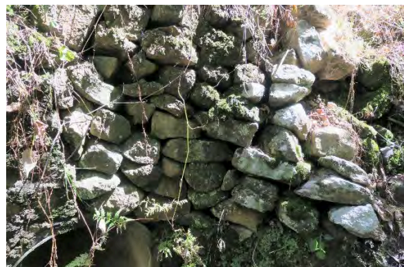
Figure 14. Site 3, detail of headwall above culvert showing dry stone construction made from irregular, uncut sandstone. Source: Extent Heritage, March 2023.
