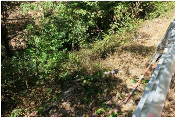
Figure 27. Site 9, embankment loss with erosion and heavy vegetation, looking south. Source: Extent Heritage, March 2023.
