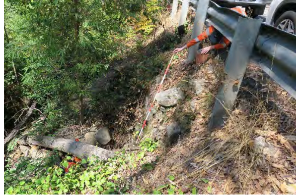
Figure 22. Site 7, eroded dry stone headwall and culvert with 2m scale, looking south. Source: Extent Heritage, March 2023.
