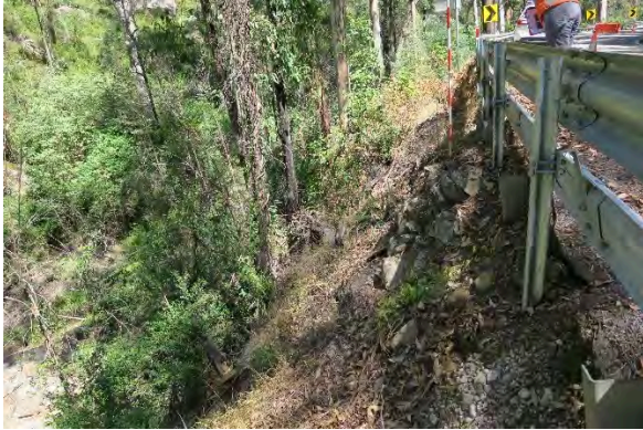
Figure 43. Site 13, dry stone wall at chainage 45-50m, erosion along embankment, looking south. Source: Extent Heritage, March 2023.
