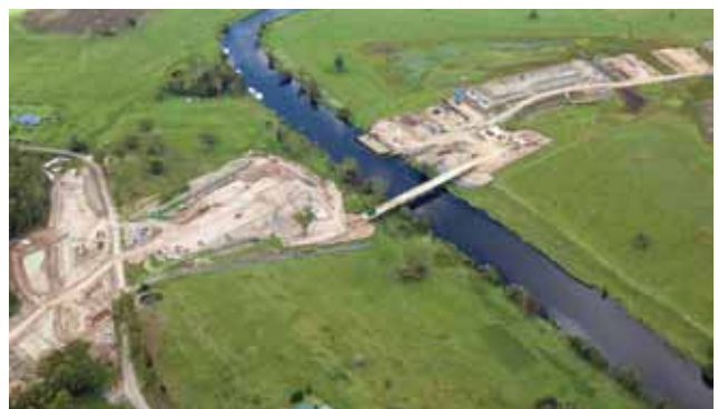
Aerial view of the temporary Myall River Bridge and new bridge works, Bulahdelah Bypass, January 2011.
