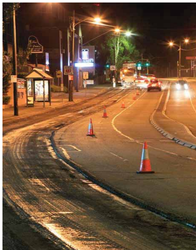
Extended right turn bay southbound into Greenwich Road on the Pacific Highway, completed under the 'pinch point' program June 2011.
