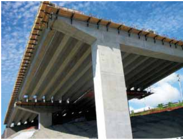
First span of super-T girders erected for the southern valley viaduct, Banora Point, May 2011.
