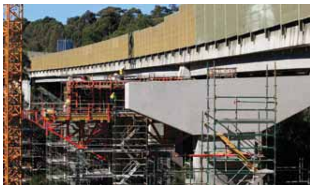
Terry's Creek upgrade, part of the M2 widening project, in construction, June 2011.
