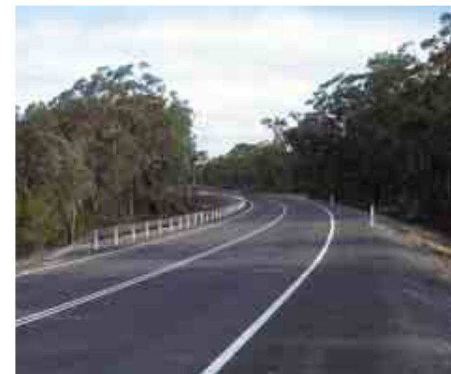
Georges Yard realignment was reconstructed as part of the Main Road 92 upgrade.
