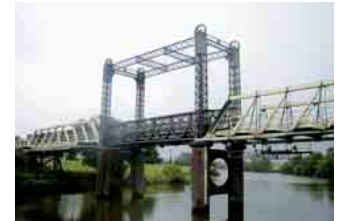
Hinton Bridge over Paterson River is an historically significant Allan truss bridge. A $9.8 million maintenance and capacity improvement program was undertaken to strengthen the trusses, approaches and lift span.
