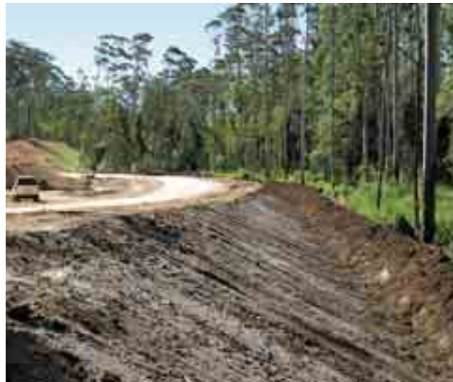
Mulch bank for sediment control along a road at Bonville on the North Coast of NSW.
