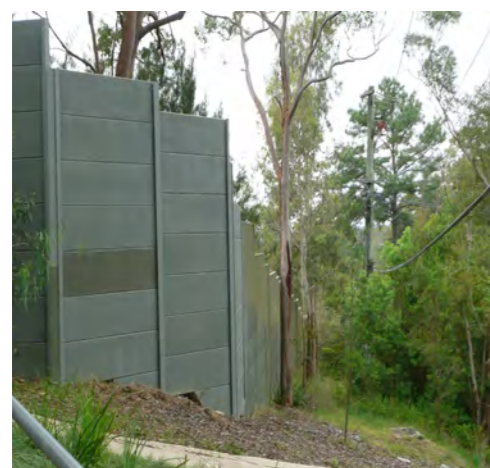
Photo 6.2.24 Existing green Hebel walls are inconsistent in colour and height
