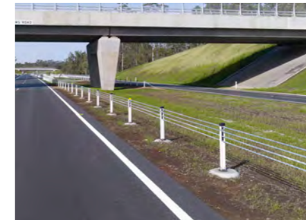
Photo 6.2.4.1 Wire Rope Barrier
