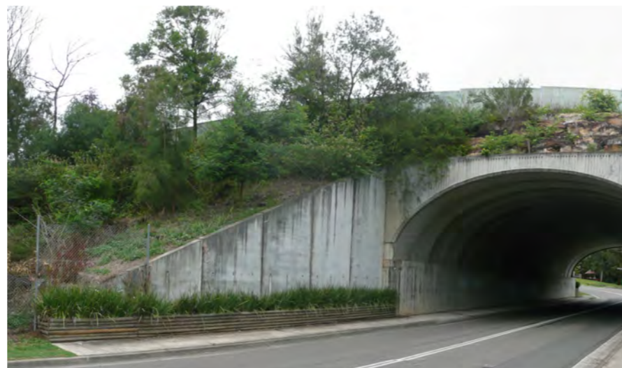
Photo 3.41 View of Busaco Road headwall, illustrating sandstone headwall, to be replaced by vertical headwall and noise wall on top.
