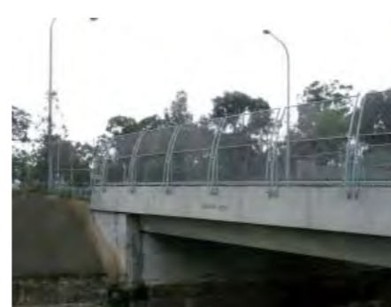
Photo 6.2.22 Existing poor quality shotcrete at abutment of Barclay Road Overbridge
