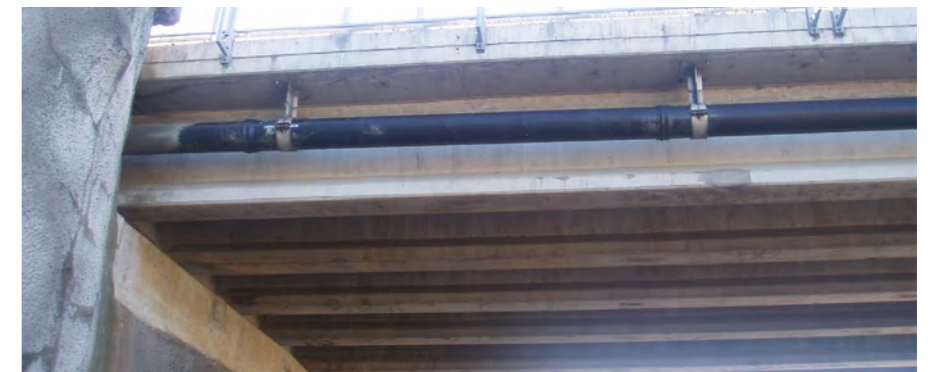
Photo 5.31 Exposed drainage pipes on Watkins Road overbridge.
