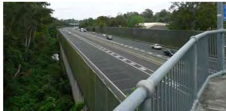
Photo 2.5 Devlins Creek runs parallel to the M2 which is constructed on a retaining wall
