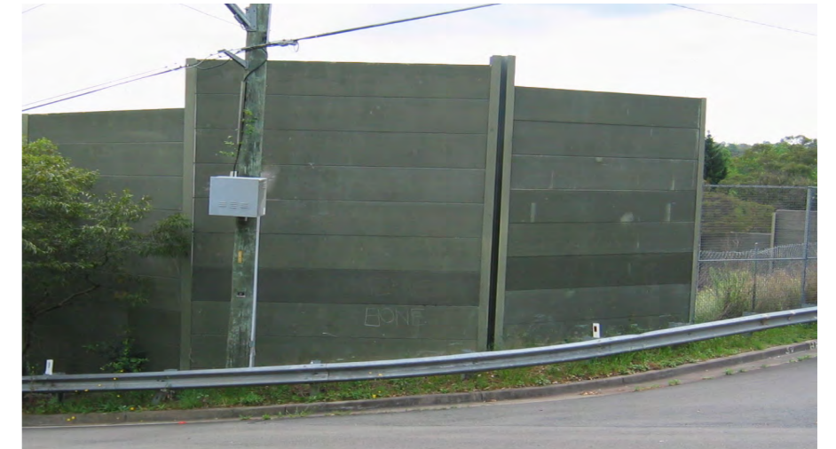
Photo 5.13 Poor noise wall termination viewed from the local road.
