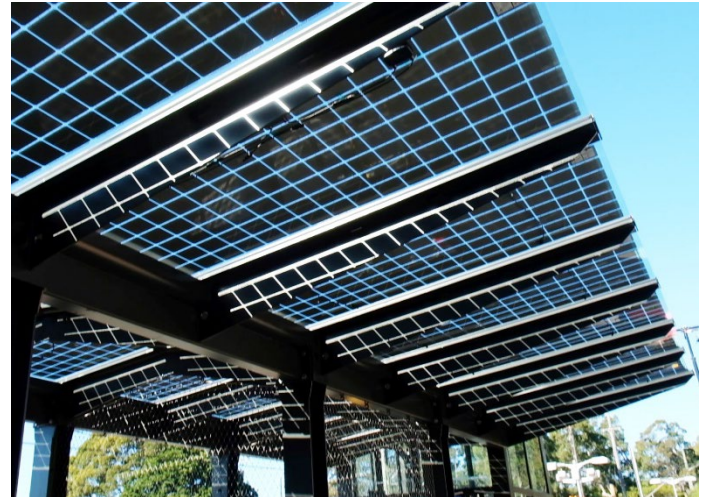
Solar photovoltaic glass installed on platform canopy
