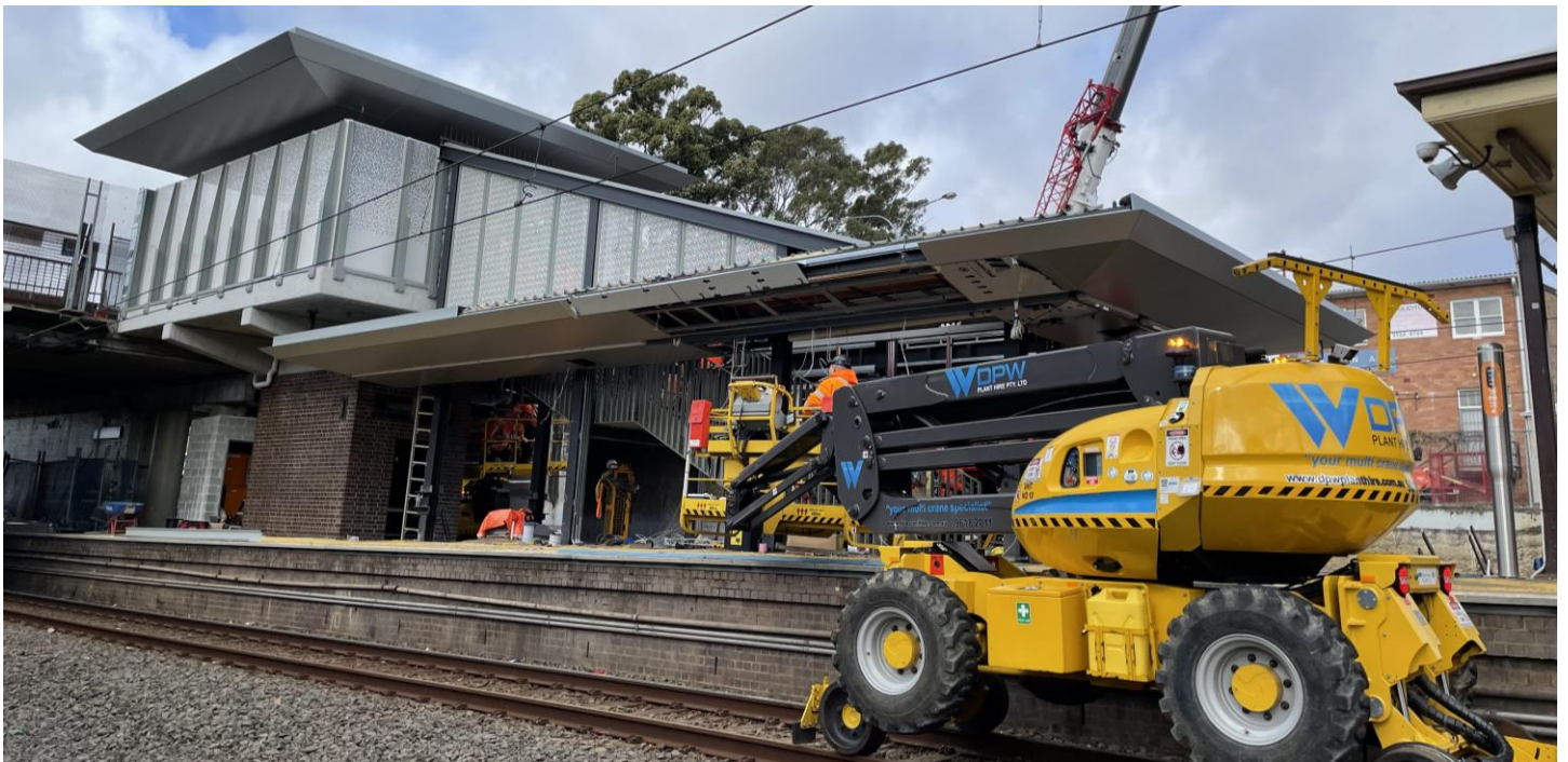
Image: The new precast concrete concourse, structural steel lift shaft and canopies were installed at Bexley North Station in June.
