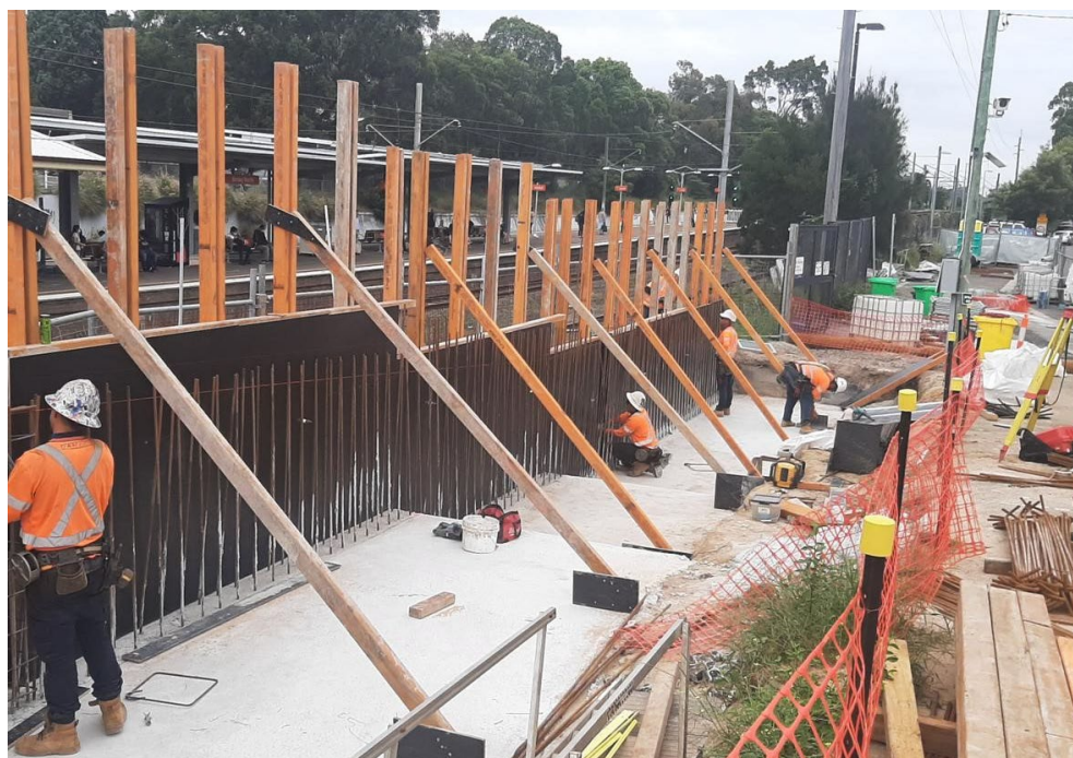
Image: Construction of the retaining wall within the Commuter Car Park, February 2021.
