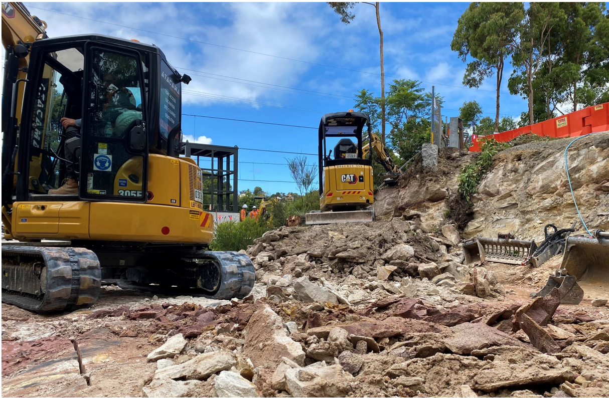
Image: Excavation underway in December for the new lift on Como Parade.
