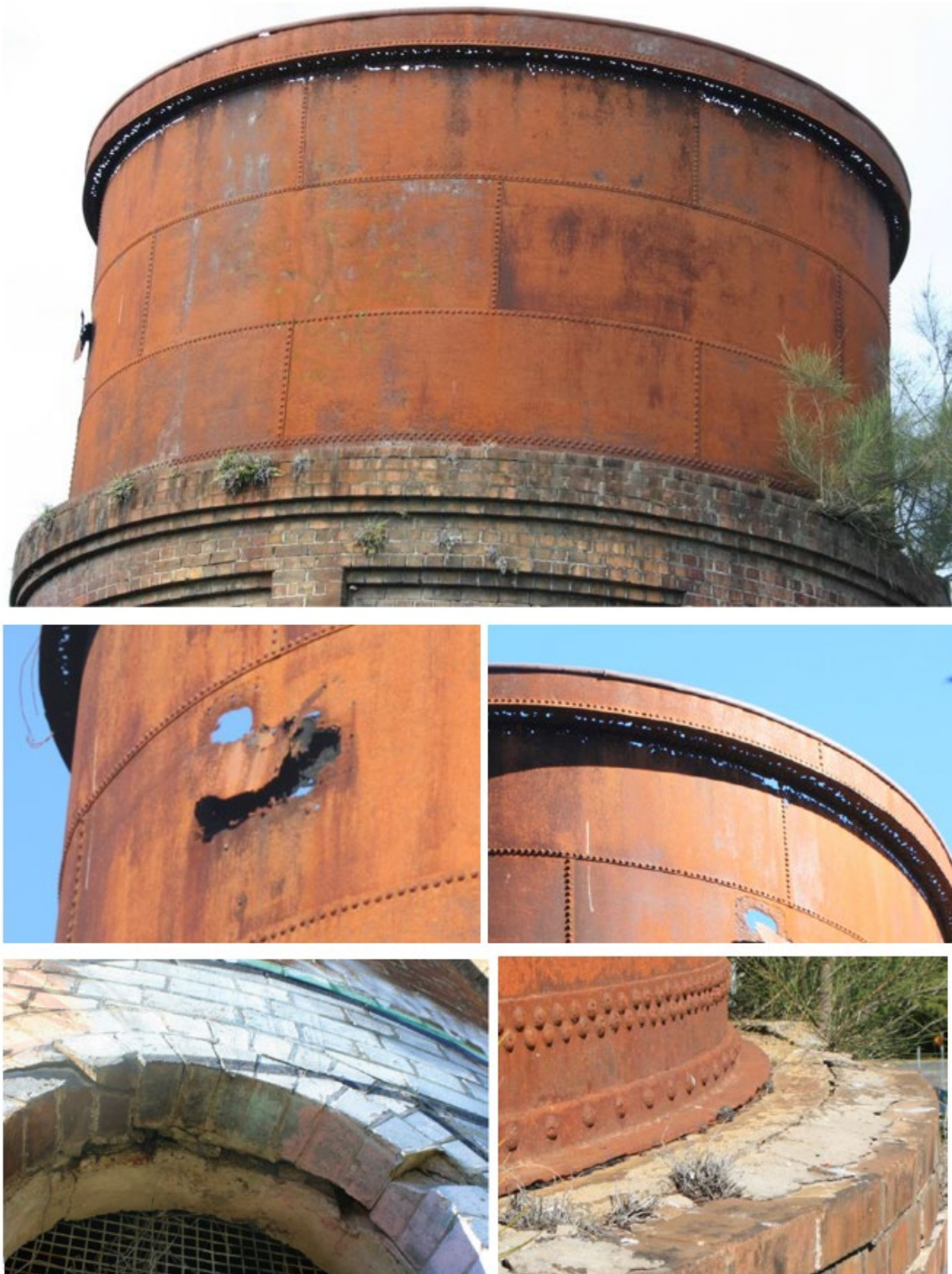
Figure 5-3: Evidence of corrosion of the upper horizontal tank and deterioration in the brick work (Extent 2018)
