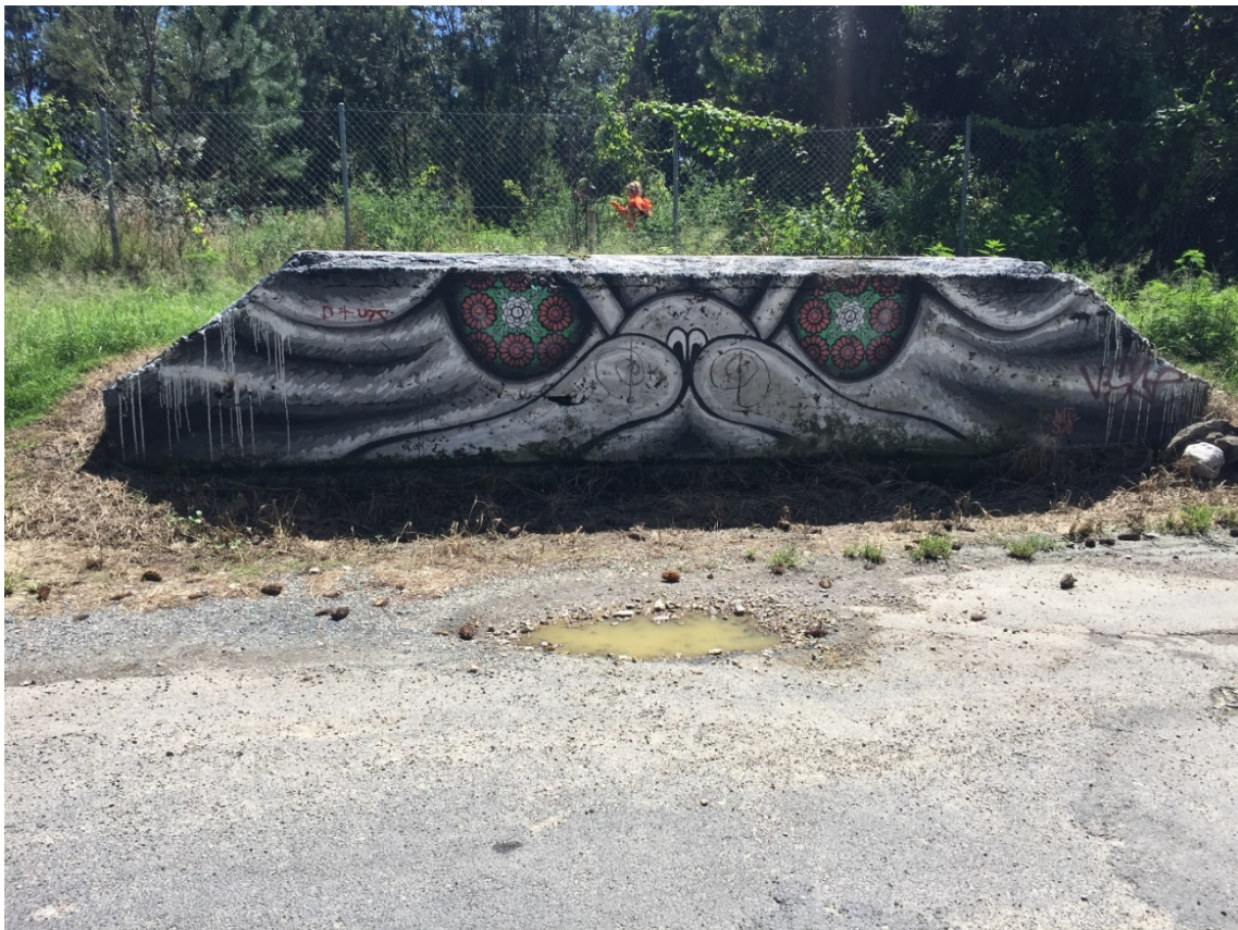
Figure 1-7: Graffiti concrete plinth along the southern boundary
