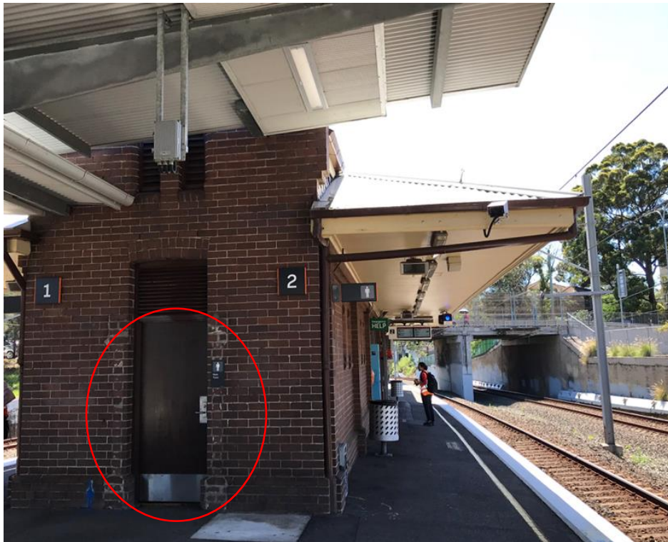
Plate 8 Western end of Railway platform building showing demolished screen walls to Male toilets.
