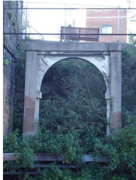
Plate 28 Trestle 1B showing extensive spalling and lack of cross bracing.
