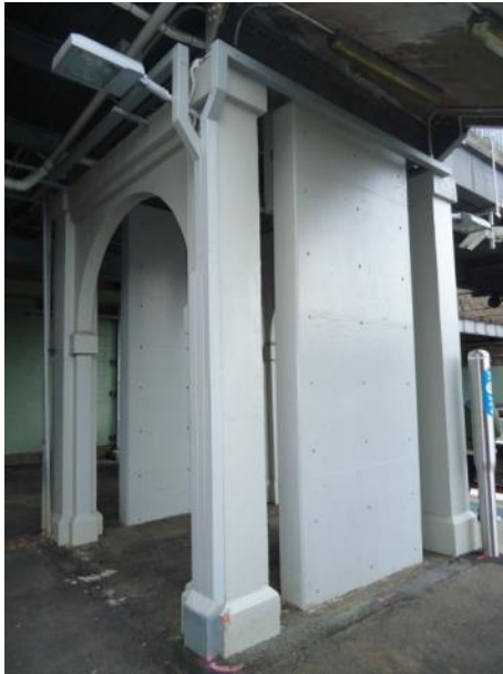
Plate 27 Trestle 4 on platform 5 showing comparative condition. Note insertion of concrete pier for 1995 overhead booking office. View north.
