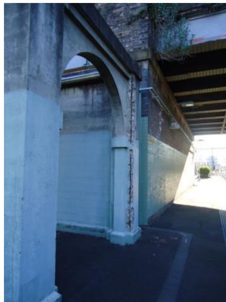
Plate 34 Detail of trestle 2A showing reinforced steel exposed for the height of the member.
