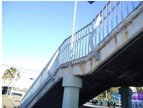
Plate 32 Stairway steel beams and balustrades on stair 3 showing general condition and form. View south.
