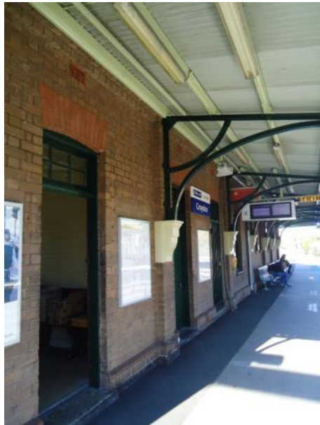
Plate 11 Platform Building 3/4 – view of western elevation showing arrangement of doors and windows
