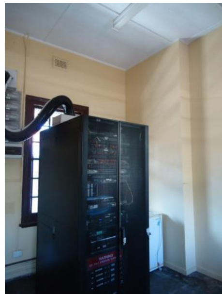
Plate 16 Platform Building 3/4 – interior of existing communications room.
