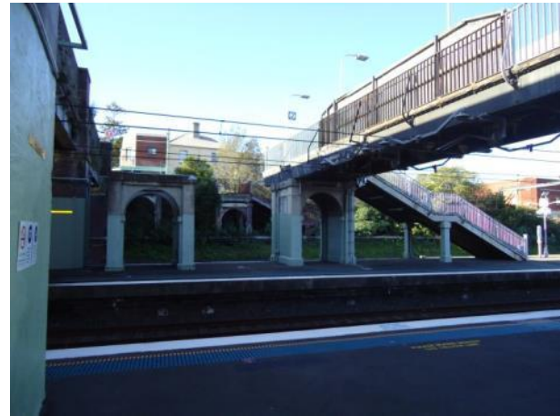
Plate 26 Footbridge span across track 4 and 5 and trestles 2A and 2B on platform 3/4.
